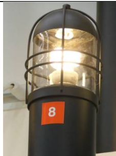
Poor – Bollard with no light control and produces glare
