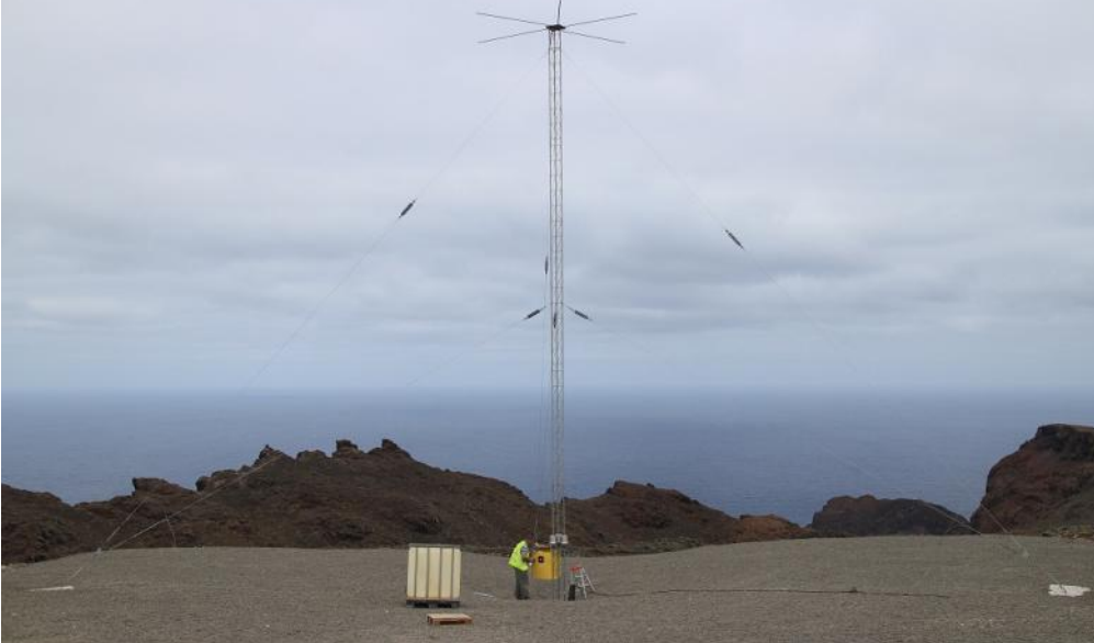
Non Directional Beacon Antenna © Halcrow
