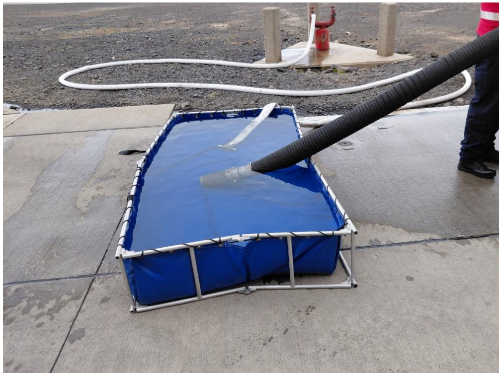
Figure 107: Opposing end of suction hose inserted into external water supply
