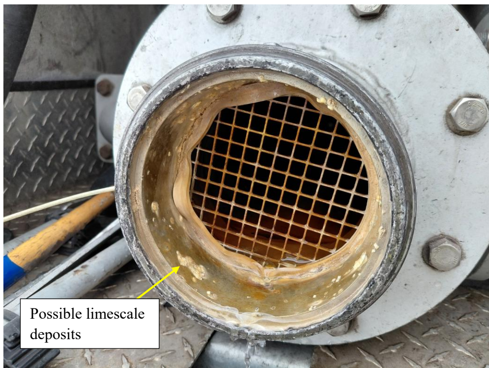
Figure 91: Limescale deposits on R1 inlet
