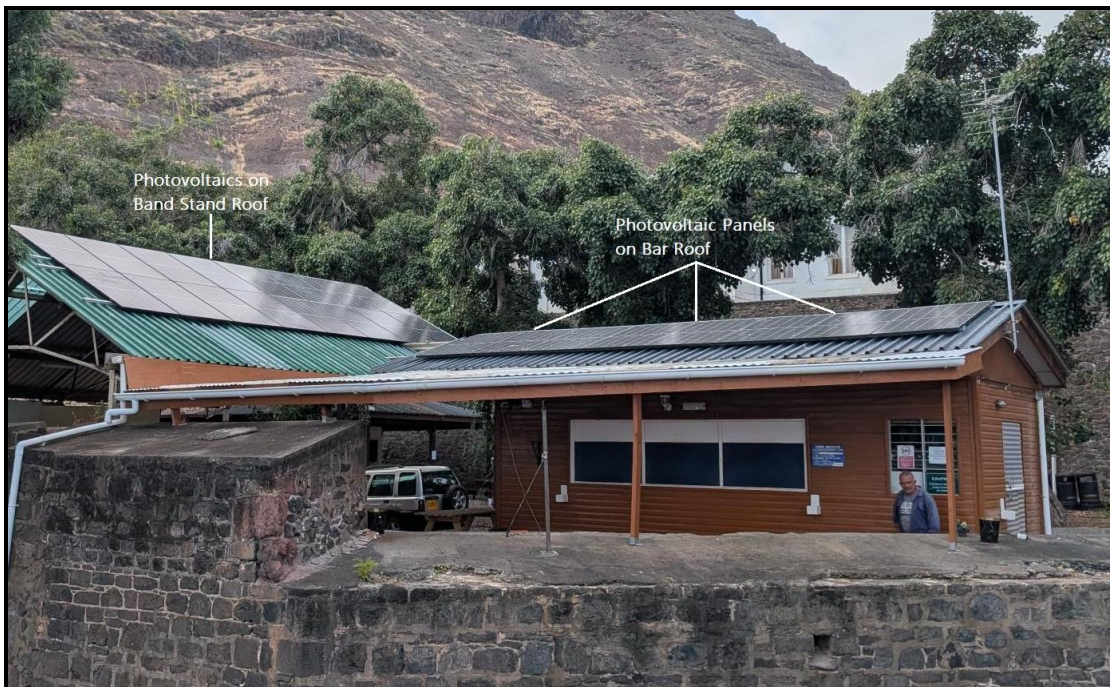
Photograph 3 – Northwest Elevation Showing Photovoltaic Panels on the Roof of the Band Stand and Bar
